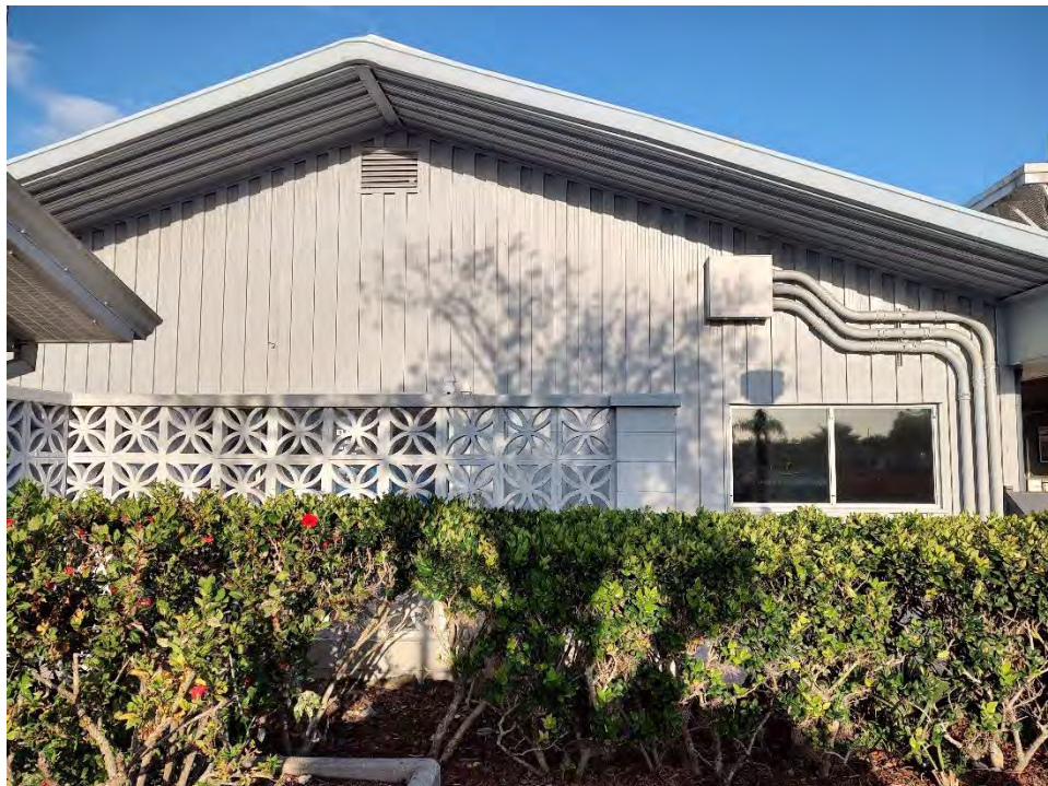
Figure 25 View west to Building 0409F breeze block wall and adjacent Building M6-0409/M6-0409C
