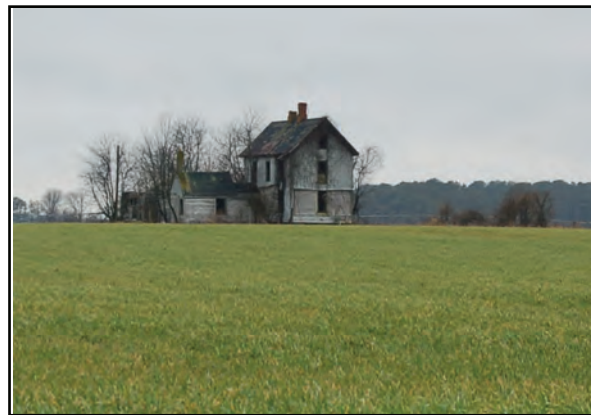
Photo 2. House at Arbuckle Neck Road does not retain integrity because of aluminum siding, removal of windows, and deteriorated condition.
