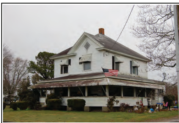
Photo 3. 12001 Atlantic Road does not retain integrity because of porch enclosure, corrugated metal awnings, and asbestos siding.
