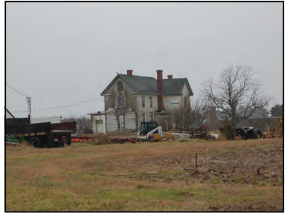
Photo 8. 32468 Taylor Farm Road does not retain integrity because of front and rear porch enclosures, porch removal, and asbestos siding.
