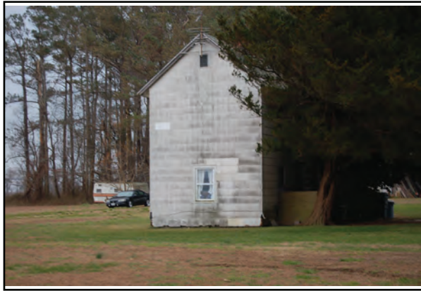
Photo 7. 31172 Pierce Taylor Road does not retain integrity because of asbestos siding, window replacement, and front addition.
