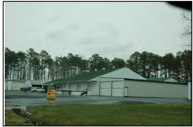
Photo 14. 31494 Wallops Island Road does not retain integrity because of aluminum siding, side addition, and garage doors and window replacement.
