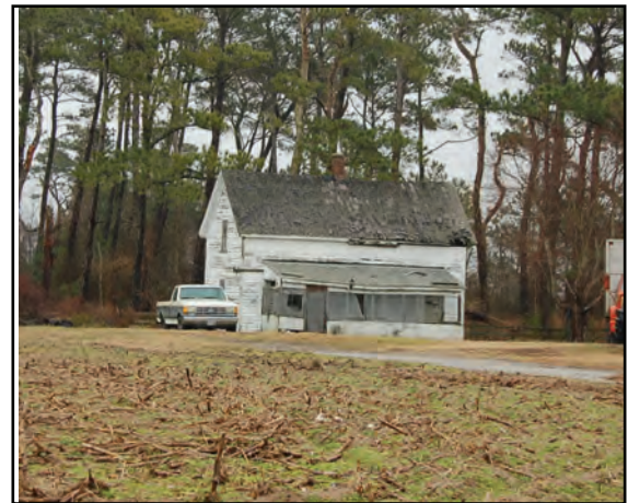
Photo 10. 33219 Taylor Farm Road does not retain integrity because of front porch enclosure and deteriorated condition.
