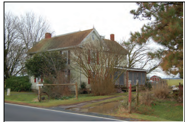
Photo 12. 32168 Wallops Island Road does not retain integrity because of vinyl siding and side addition.
