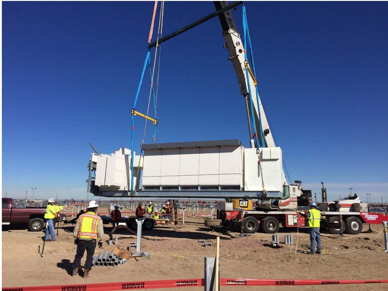
Figure 5 Pre-Assembled Power Conversion Station on a Steel Skid
