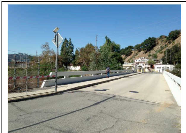
The NASA JPL Bridge provides vehicular and pedestrian access to the East Gate at NASA JPL.
